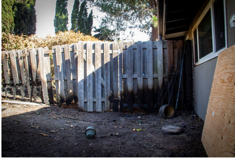
Figure B4.2. Photograph of a fence, following the 2024 Mountain Fire in Camarillo, CA, which had ignited adjacent to a home where fire spread to the wall of the structure. In this case fire service intervention and the presence of noncombustible wall cladding (stucco) helped avoid ignition of the structure. The window frame on the right side of the image was damaged, and there was evidence of sufficient radiant heat to damage the paint in the eaves of this home. Photograph by Evan Sluder.
